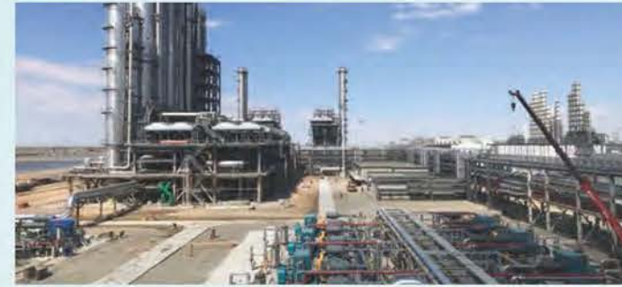
东方希望多晶硅项目 Project of Polysilicon for East Hope Group
