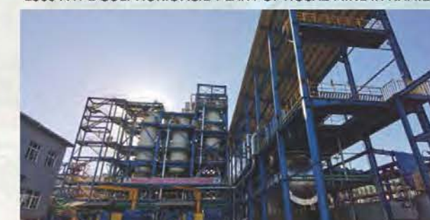
印尼OBI红土镍矿湿法冶炼项目 Project of Nickel Laterite Hydrometallurgy of OBI in Indonesia
